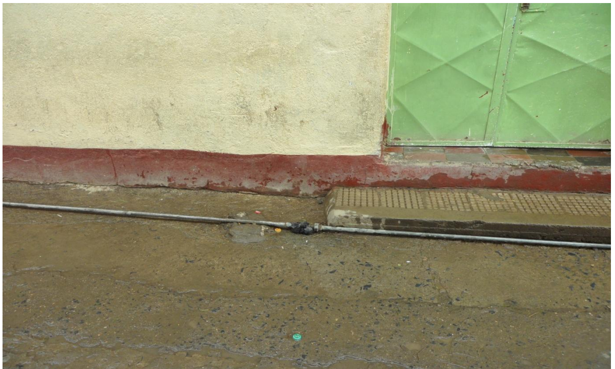
Figure 10: Leakage Case Reported After 24 Hours
