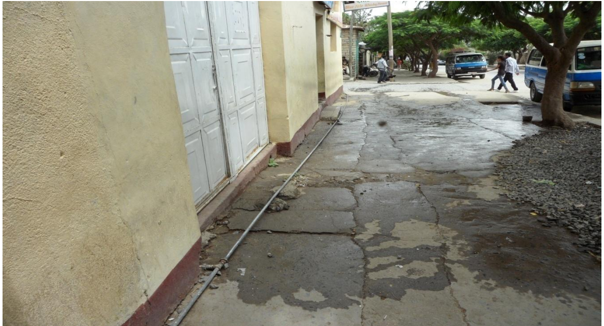
Figure 8: Water Leakage in the Old Sub City of Mekell
